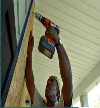
Board up windows or attach storm shutters.
